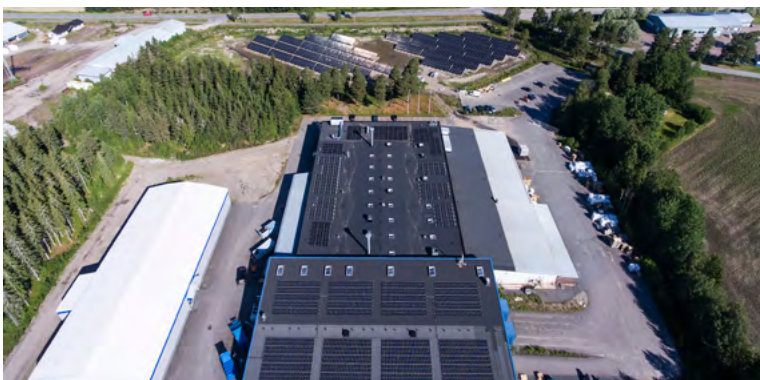
Solar park and solar installation on the roof at Coreplast Laitila Oy.
