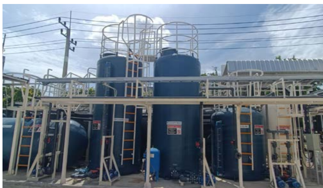
Wastewater treatment plant installed at STT
