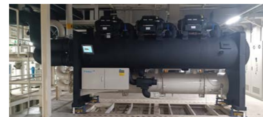
Chiller system installed at STT
